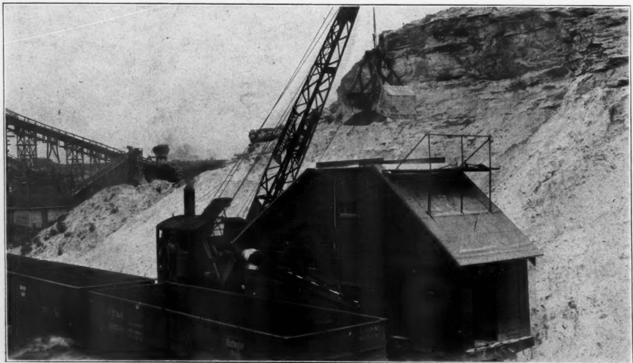
View Showing Crane and Portable Car Which Carries the Screening and Crushing Apparatus and Discharges the Moulding Sand into Car Alongside
